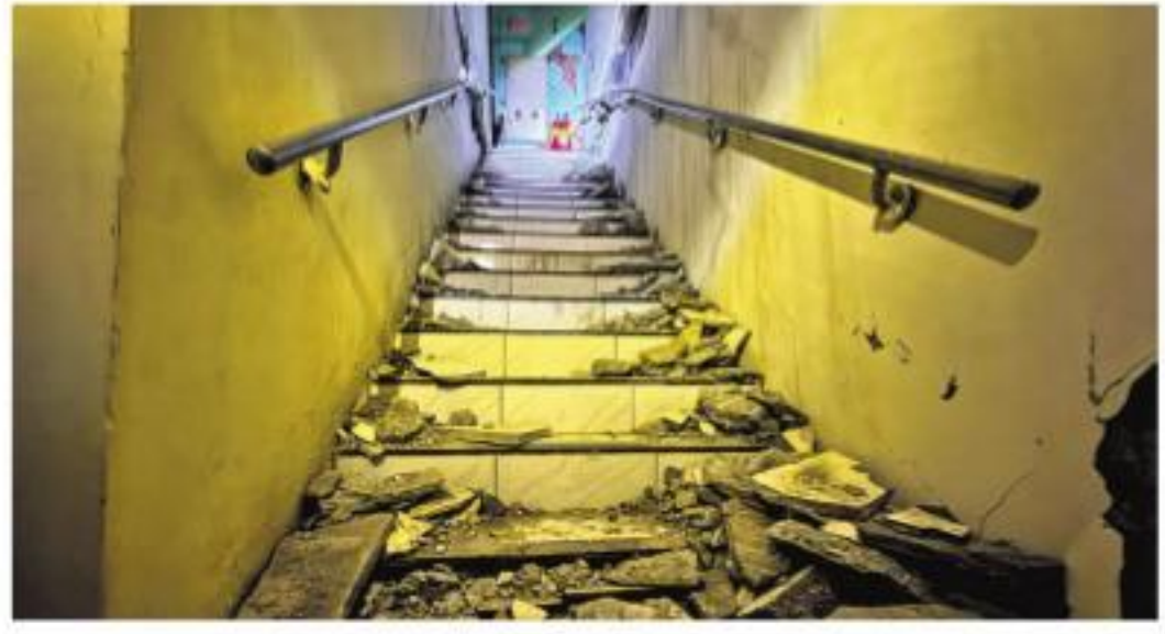
Debris is seen along a staircase of an apartment building damaged in Wednesday's earthquake, in Taiwan's Hualien County | AFP
